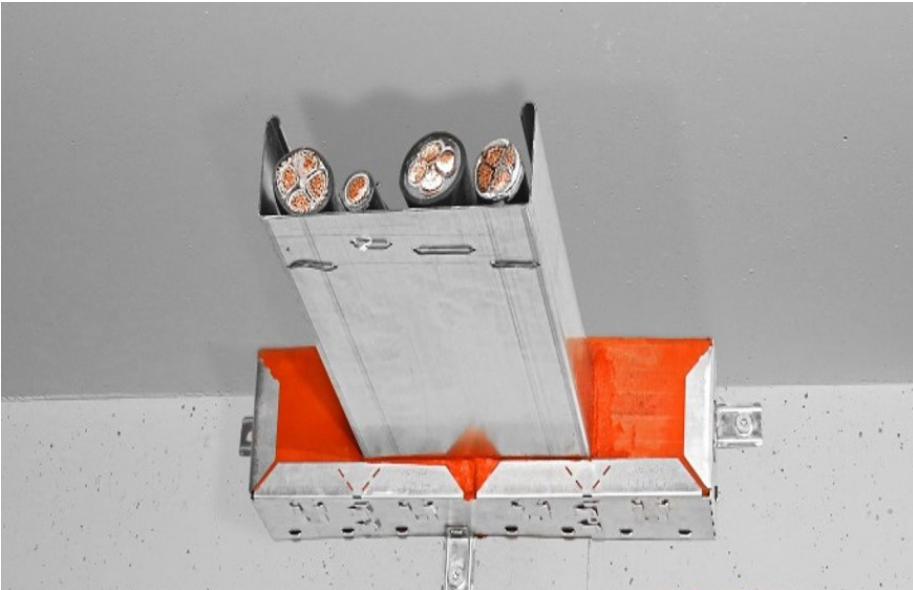
(a) Lack of firestop sealant to enclose firestopping of multiple penetration, i.e. cable tray and cable bundles, and barrier
