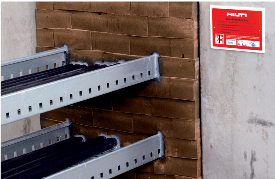
Figure 5.4 Marking and identification of firestop assemblies
